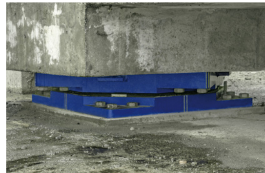
Installed SIP®-D-Bearing under a pier of the Yarumo Blanco Viaduct in Colombia.
