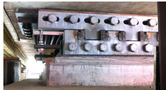
Installed bearing. During the construction phase in the launching process, temporary restraints had enabled the bearings to partly assume changing functions in the progress of construction work.
