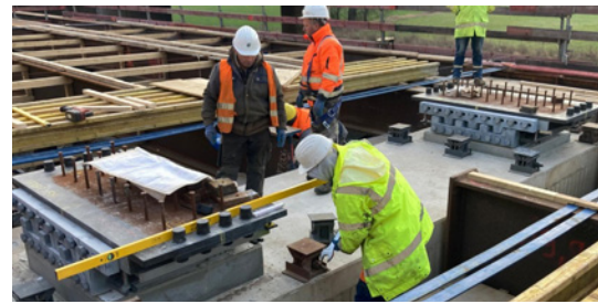
Installation of the bearings on the first new section of the Leverkusen Bridge.
