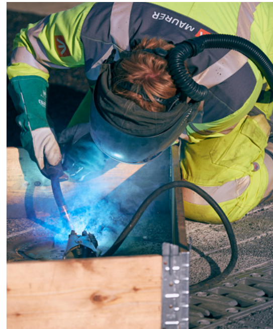
Fine-tuning. Visible front right: the roadway expansion joint integrated in the Mega-MMBS.
