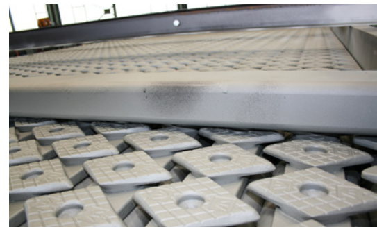
Detail: Noise protection in the form of welded rhomboid plates. Welded rhomboid plates are more stable under traffic than bolted solutions.
