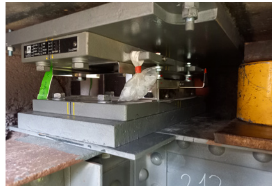
...and the situation is no better at the upper bearing.
