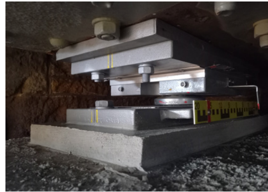
No more space was available: extremely tight spatial conditions at a bearing under a steel girder...
