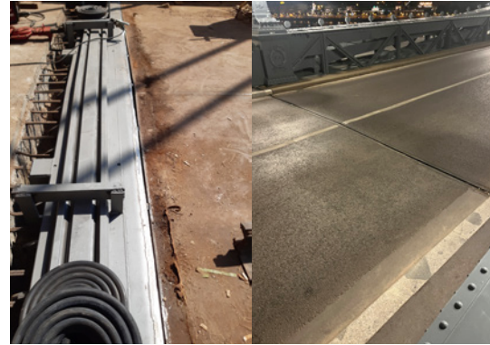
Installation of an expansion joint at the renovated bridge ends – on the right an installed expansion joint. Photo: MAURER
