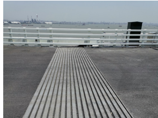
The expansion joints at the Hutong Bridge north of Shanghai feature a length of 36 m each.
