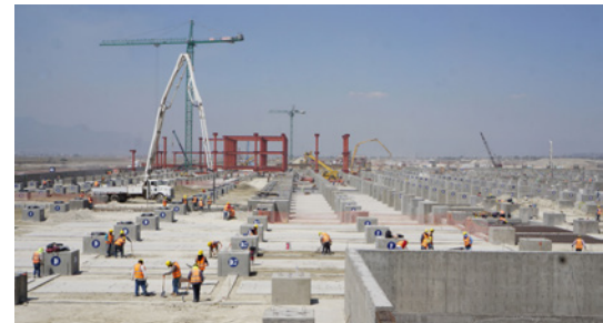
The entire terminal will be resting on seismic isolators.
