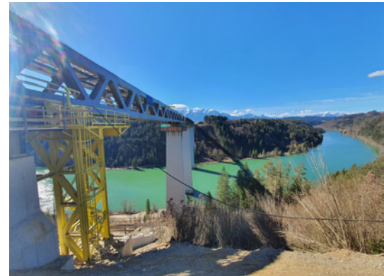
Jauntal Bridge over the Drava River during the launching process in March 2023. The old bridge deck is darkly visible in the centre of the picture.
