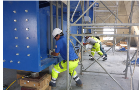
Four workers move the 400-t mass block to measure the pendulum frequency.
