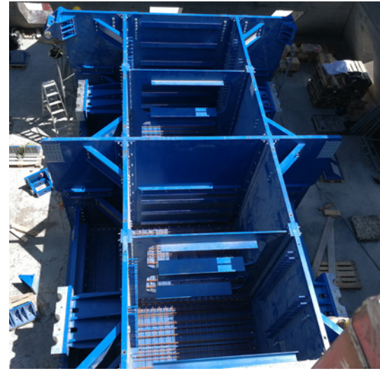
View from the tower top into the chambers of the steel box. At the bottom, the steel reinforcement of the concrete can be seen: in total, 220 t were filled in.
