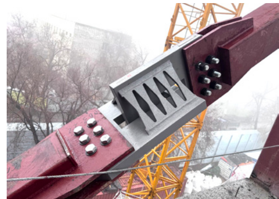
A SHARK® with 2,400 kN of response force installed in Almaty.
