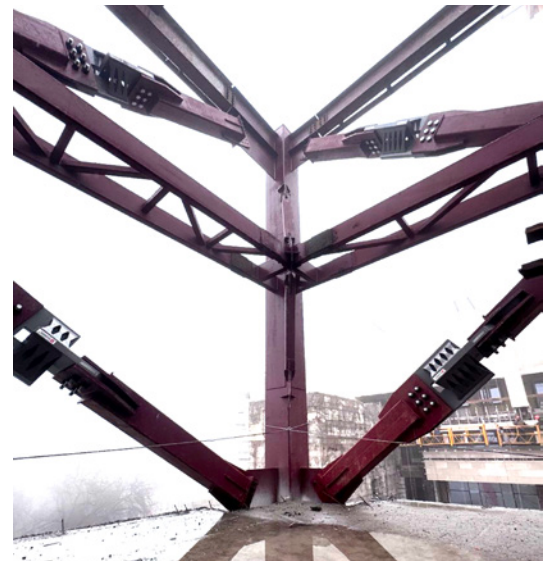
Four SHARKS® at the corners of the two top floors. On the right are SHARK® 2400 kN and on the left are SHARK® 1400 kN.
