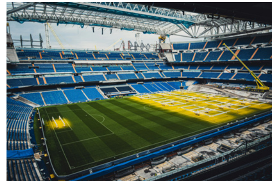
The Bernabéu during construction. The bearings, each with a load-bearing capacity of 67 MN, are fitted at the outer corners of the roof structure (at the rear of the image).
