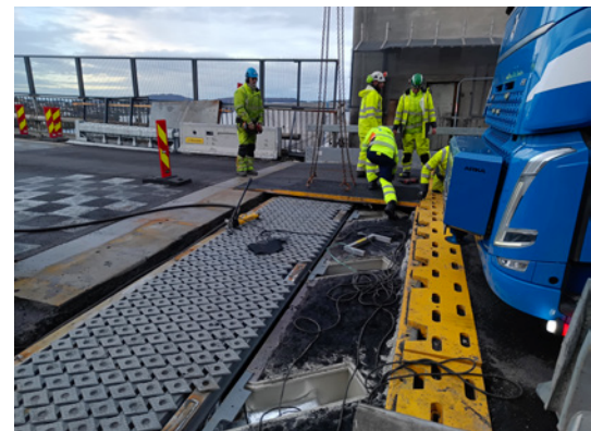
The installed centre beam box, with the steel connection on the left and the old, but also renovated joist box on the right.
