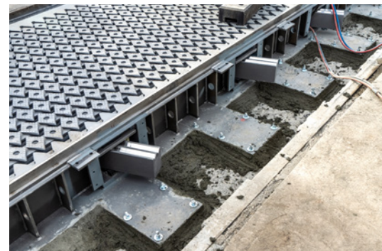
The expansion joint after installation. This image shows the joists with the gleaming W-shaped catamaran supports. These support the profiles running transverse to the road direction, with the rhomboid plates for noise reduction on top.
