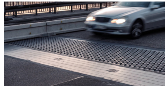
The installed expansion joint with traffic passing over. The rhomboid plates reduce the noise of the vehicles.
