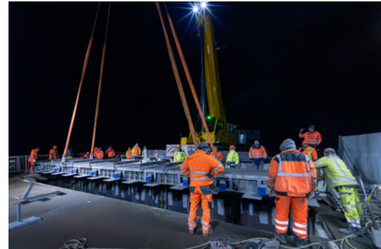
The new, 12-profile expansion joint is installed on the Saturday night: a complex operation that called for a large team of specialists.
