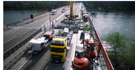
The image shows the new expansion joint on the left, which was replaced on the previous weekend, under traffic load. On the right is the gap following the removal of the old roller shutter joint.
