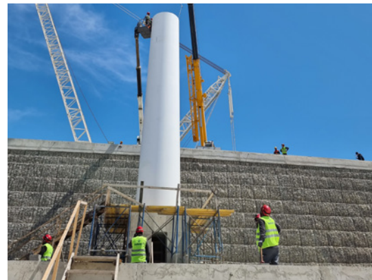
The tuned mass dampers were gradually inserted and installed in segment 9 of the flagpole, before the complete segment was mounted on the mast. Photo: MAURER
