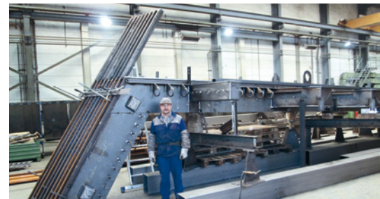
3 m high and at their end being executed watertight: the edge structures of the Stadsbrug at the manufacturing site in Munich.
