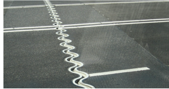
The first wave joints in the Netherlands at the Stadsbrug in Nijmegen.
