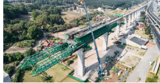
Construction site of the new intercity line connecting Toluca and Mexico City.
