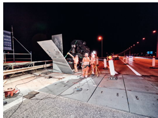
A fast and simple process: opening and closing of the modular job site bridging system by way of a linkage.
