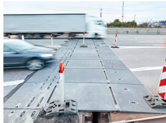
Traffic is still flowing: the MMBS steel plates can be passed at up to 70 km/h. Below to the left the structural gap can be seen, with the old expansion joint already removed.
