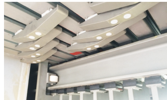
The new design of the control system of the sliding lamella expansion joints.
