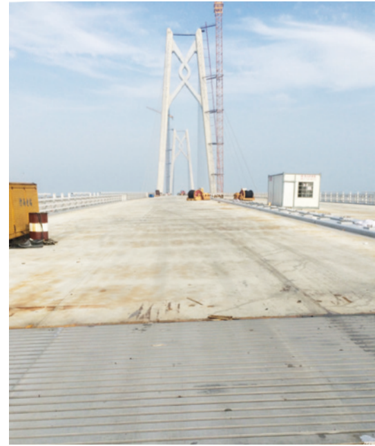
The new sliding-lamella expansion joints were inserted at the main segments of the Jianghai cable stayed bridge.
