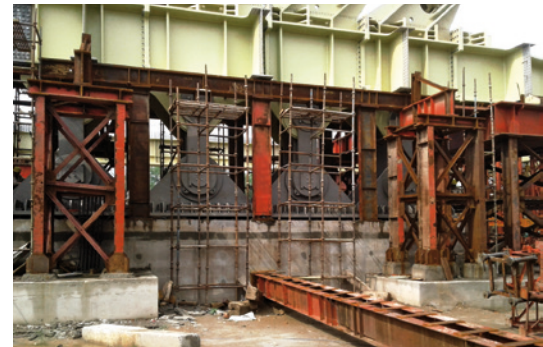
The pendulum bearings (gray) accommodate the tensile forces of the backstay cables (anchoring visible at the upper right of the picture) and allow for longitudinal movement of the bridge deck (lime green).
