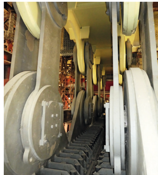
The pairs of pendulum bearings viewed in longitudinal direction of the bridge. At the outside the two steel mounting plates, top and bottom: rod ends with axial pivotal bearings.
