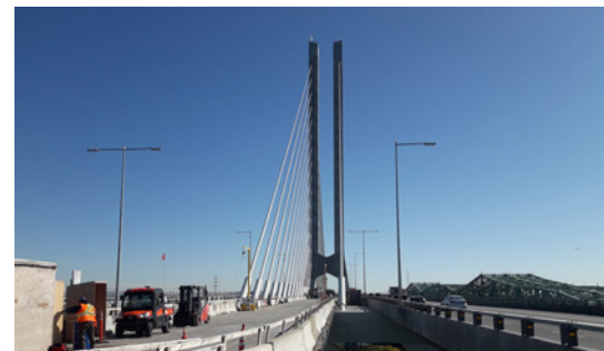
The central bridge, a railway bridge, under construction. It passes through in between the characteristic towers of the New Champlain Bridge. On the right, four-lane road traffic has already been flowing for three years.
