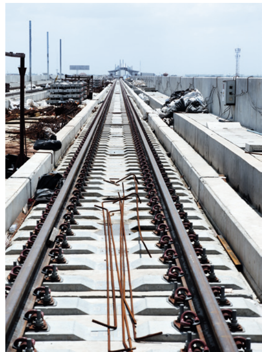
The 'Red Line' features two tracks per viaduct with a track gauge of 1 m.
