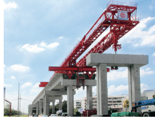
The 'Red Line' is designed as an elevated railroad on 22 m high viaducts. Each direction of traffic has its own viaduct with two tracks.
