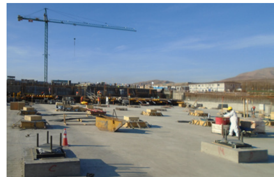
Foundation of the clinic centre in Alto Hospicio in 2019: On top of the concrete bases lie the first SIP®-D-Bearings.
