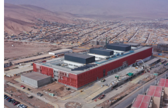
The clinic centre in Alto Hospicio in May 2021. The building structure is in place – entirely seismically isolated.
