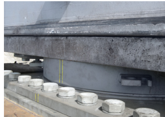
The bearings underneath the Bogibeel Bridge transmit a load of 2,800 t in the smallest of spaces.
