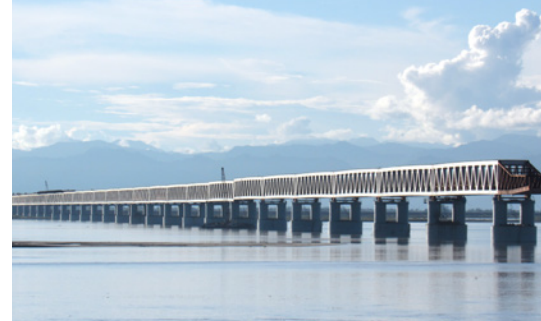
The Bogibeel Bridge across the Brahmaputra, at the bottom of the Himalaya. The picture was taken during construction in 2017.
