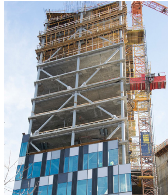
The building in 2017. Clearly visible are the diagonal braces of the outer steel structure, each spanning across two stories.
