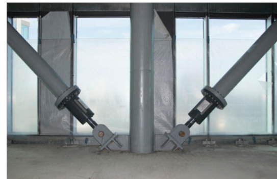
The dampers with a length of 750 mm are installed at the bottom end of the cross braces.
