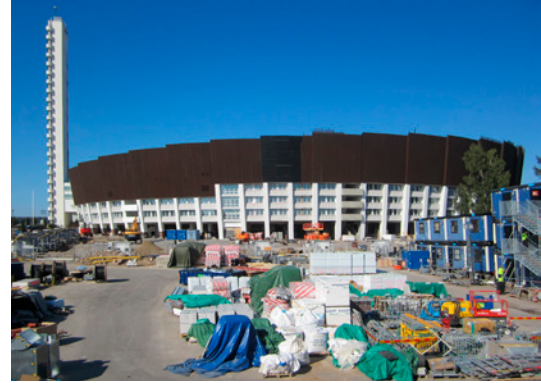
Helsinki Olympic Stadium with building site storage in front of the listed and renovated façade.
