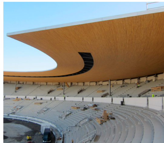
The renovated stands with the new roof. The steel supports in the seating rows carry the main load. Underneath the roof, the 84 smaller bearings are positioned that mainly accommodate the tensile load caused by the weight of the cantilevered roof.
