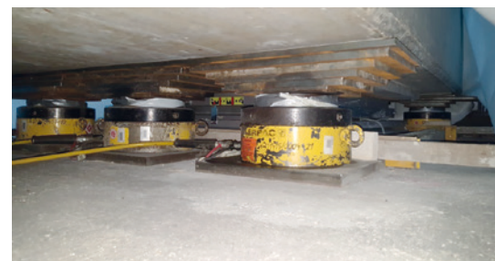
Extremely constrained spatial conditions occurred at Pier P7 of the Reichsbrücke in Vienna, where the structural bearings had to be replaced.
