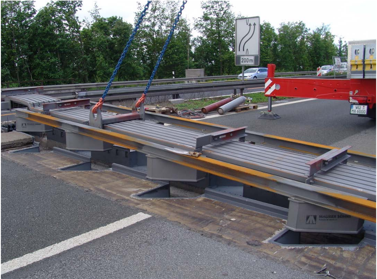
MAURER Expansion Joint Retrofit System „Box-In-Box“ - lifting the new expansion joint into the old and prepared block-out
